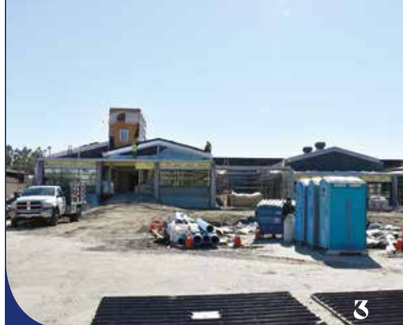
February 7, 2019, windows have been installed and the new Center is beginning to take its final form.
